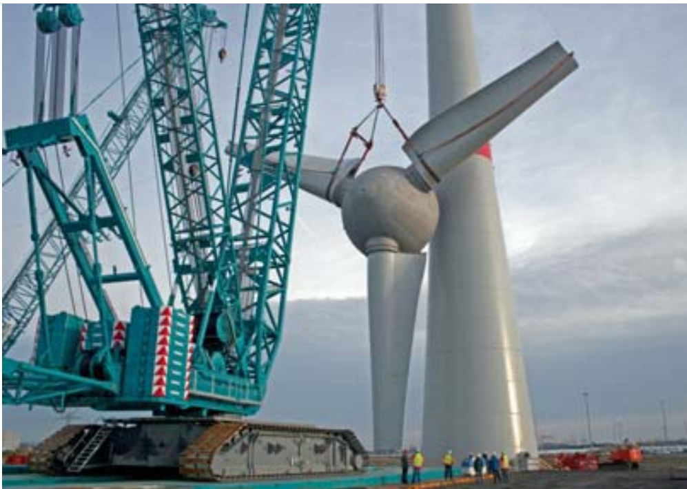
Figure 1. Lifting of the 340 t hub section for Enercon E-126 7,5 MW wind turbine. The Terex Demag CC9800 crawler crane is formally rated 1600 t and in this configuration can lift 360 t.
