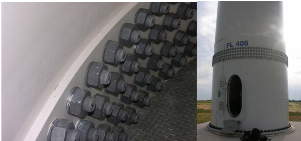
Figure 6. Screw joint in the tower of a Fuhrländer 2,5 MW in Celle, Germany.
