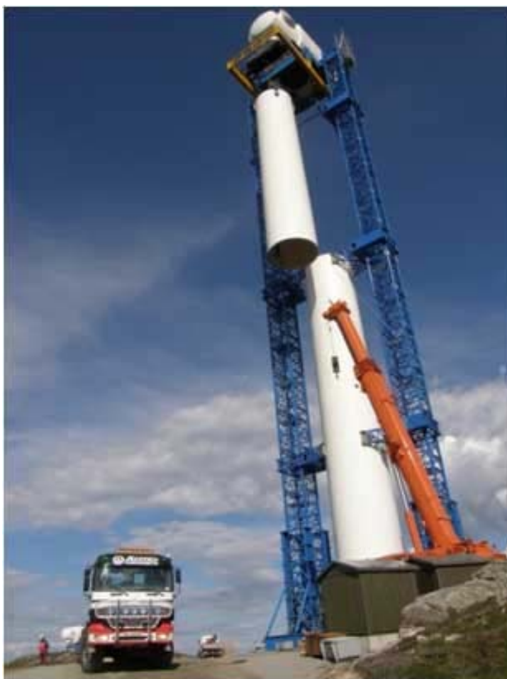
Figure 2. Lifting towers in use for assembly of Scanwind 3 MW wind turbine at Hundhammerfjell, Norway. Lifting operation performed by Sarens Transrig AS. Note that the wind turbine tower is used for stabilizing the lifting towers and that a small mobile crane is used for assisting lifts.
