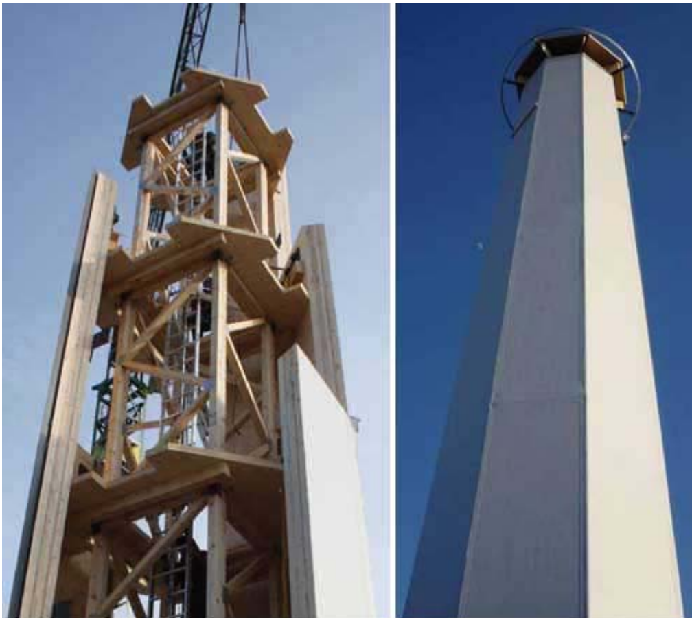
Figure 22. A wooden tower built by Timber Tower, Germany, 34 for a Vensys 1,5 MW wind turbine. Left a wooden panel lifted during the assembly, right the tower finished.
